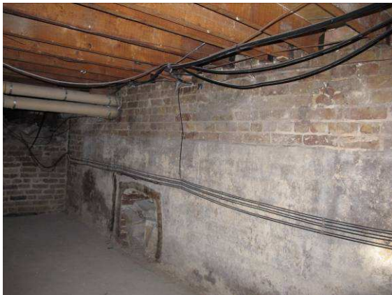
Photo from basement showing existing timber floor structure. All manifolds were located here.
