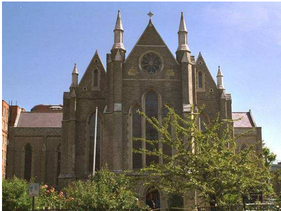
As part of the reordering of the Church Of Our Lady, a new floor incorporating underfloor heating was installed.
