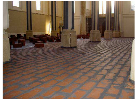
Shot showing the JUPITER Screed Replacement Tiles installed before the final floor tiles were installed. A ramp from the main entrance was formed to cater for the increase in floor height.
